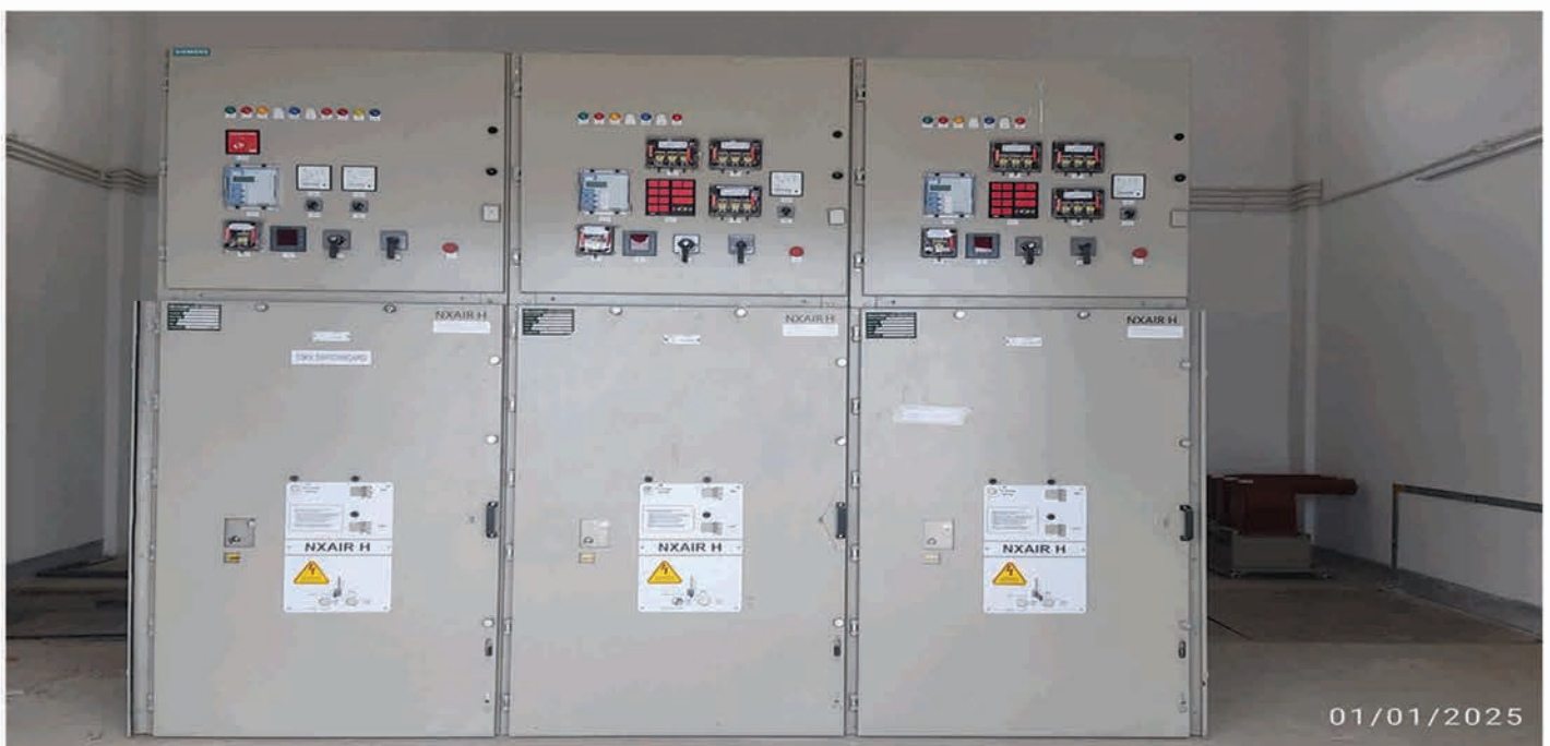
HIDCO 33KV Sub-Station, New Town
