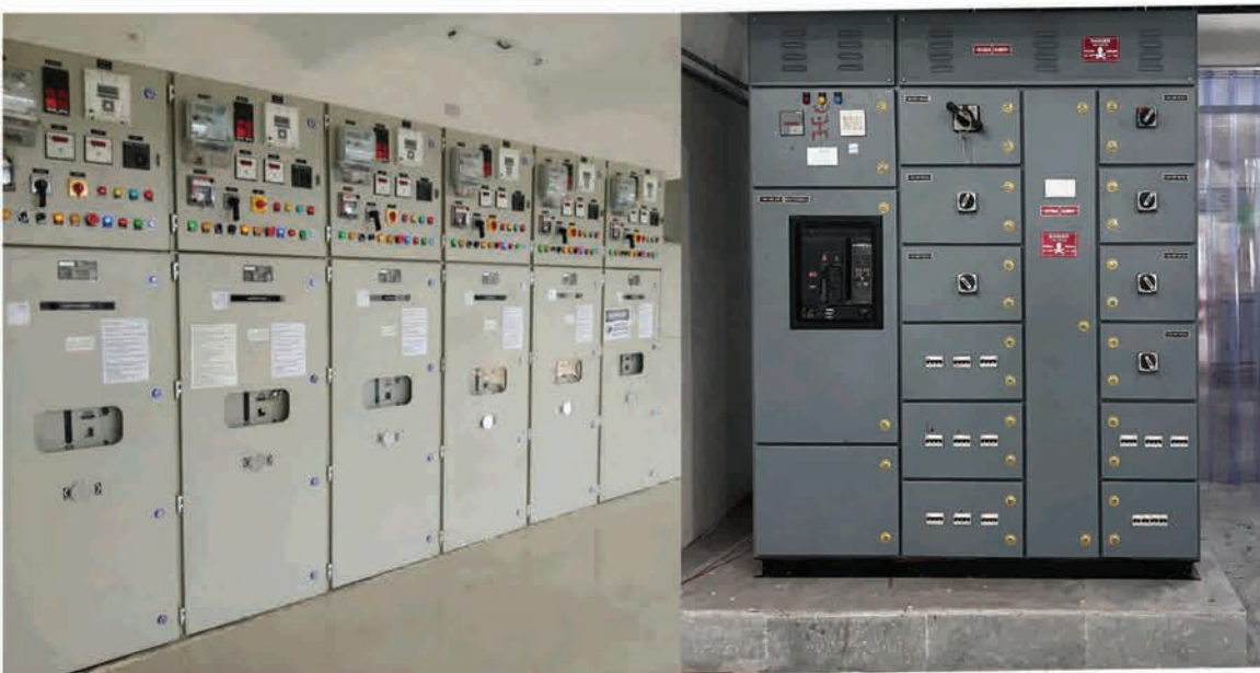
Switchgear Panel for Steel Plant
