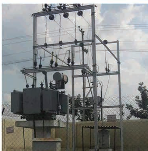
33kV transformer commissioning
